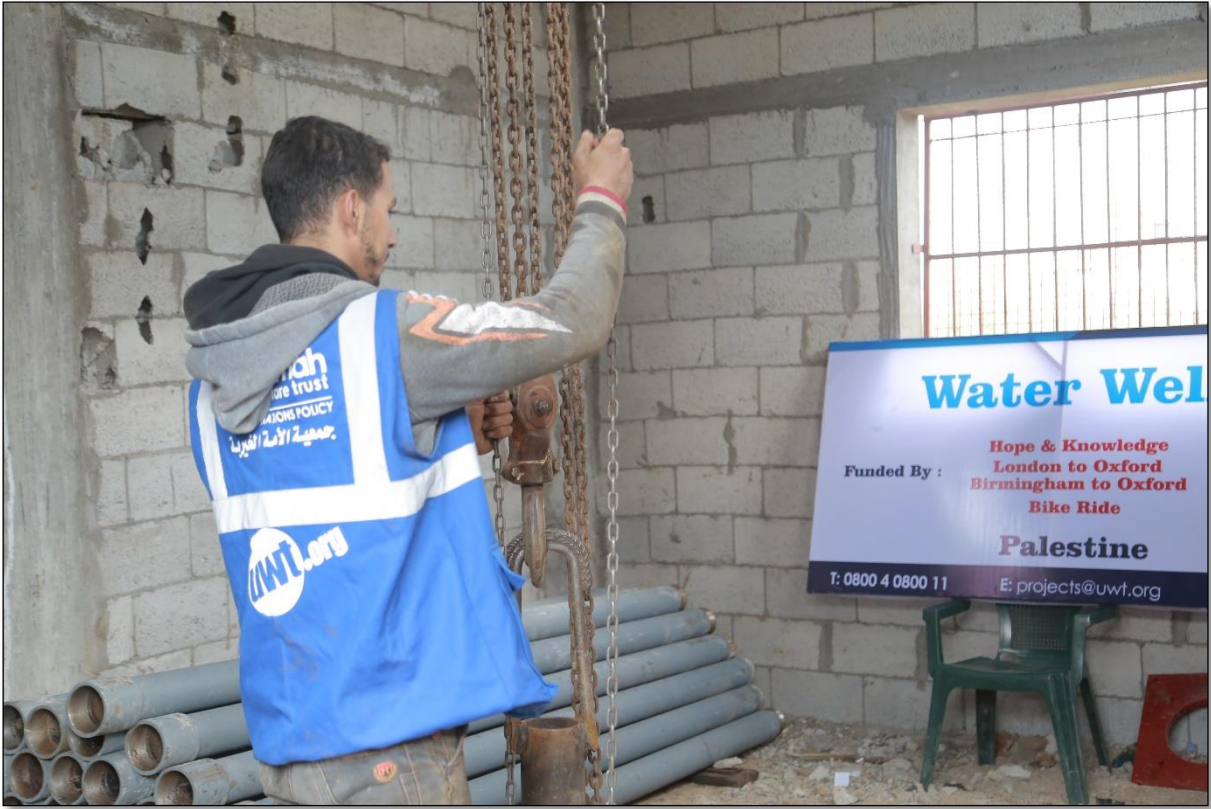
Water Pumping Unit Has Been Installed
