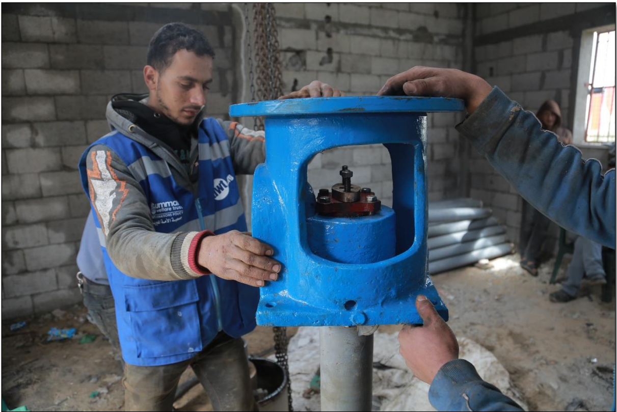
Electrical works, UPVC pipes & Connection with water network is now remaining to be installed
