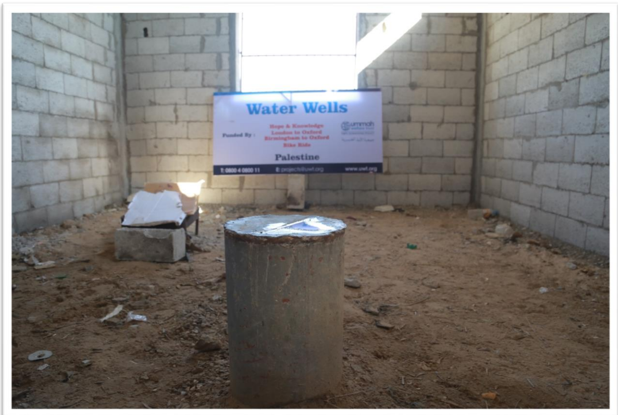
Water pumping unit, chlorine disinfection system and electrical works are now remaining to be installed.
